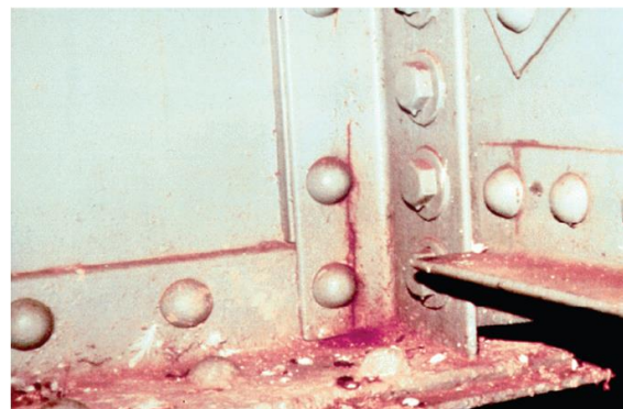
Cracked Stringer to Floorbeam Connection Angle
