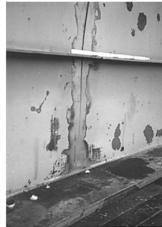
Crack in Girder Web from Splice in Longitudinal Stiffener
