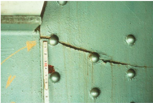
Fatigue Crack at Coped Top Flange of Riveted Connection
